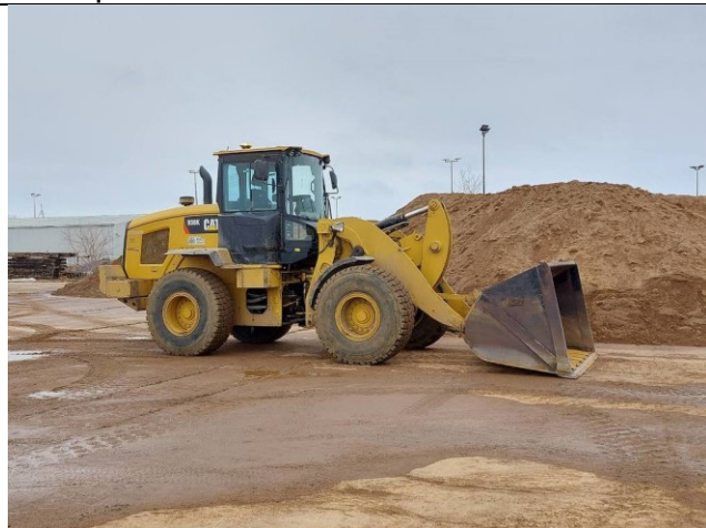
Caterpillar 938K Loader Used as a chase loader, cleaning corners and cul-de-sacs
