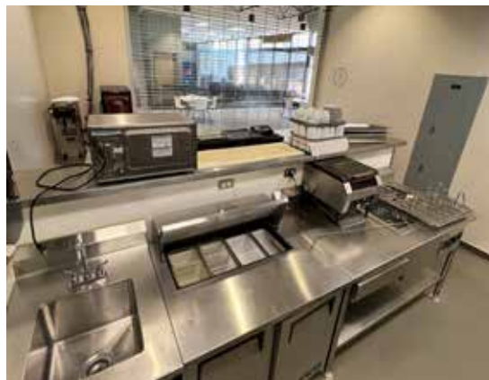
(Above) Commercial kitchen & cafe area failed and has remained closed for the past 5 years. (4) Vending machines & coffee service these areas adequately.
