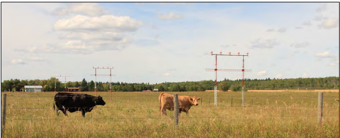
Runway 08 SSALR Approach Lighting
