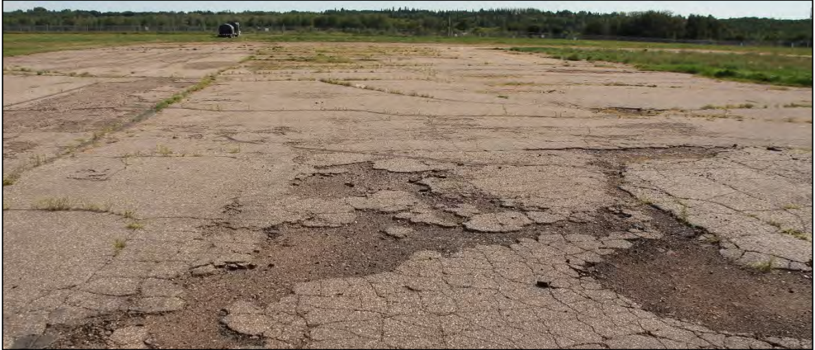
Apron II pavement distresses
