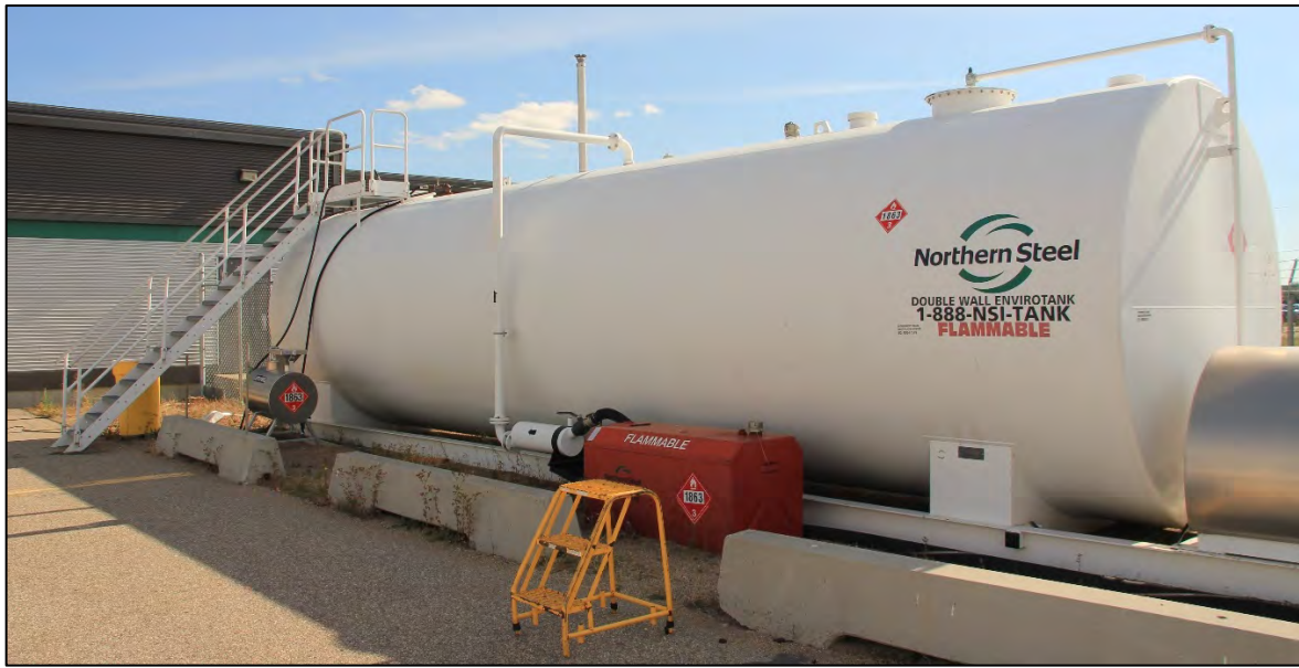
77,000 L Jet-A tank adjacent to the terminal building
