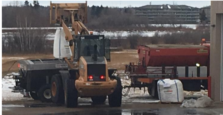
2006 Case Loader loading granular de-icer into the 2015 Spreader towed by the 1989 Navstar de-icer truck.
